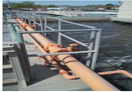
Aerated Grit Chamber
