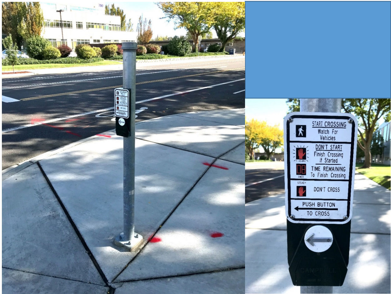
Figure 2- 7 - Pedestrian activated push button
