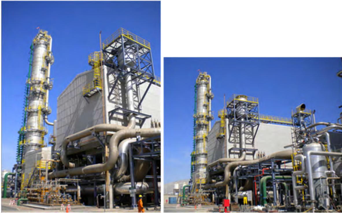
Figure.5. Example of shelter for Nitric acid outdoor.
