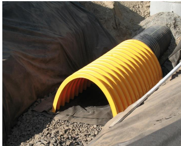
Installation of a commercially manufactured stormwater infiltration device which meets the definition of a UIC well
