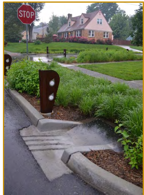
Example photo of a curb cut inlet into a bioretention facility (not the preferred approach.)
